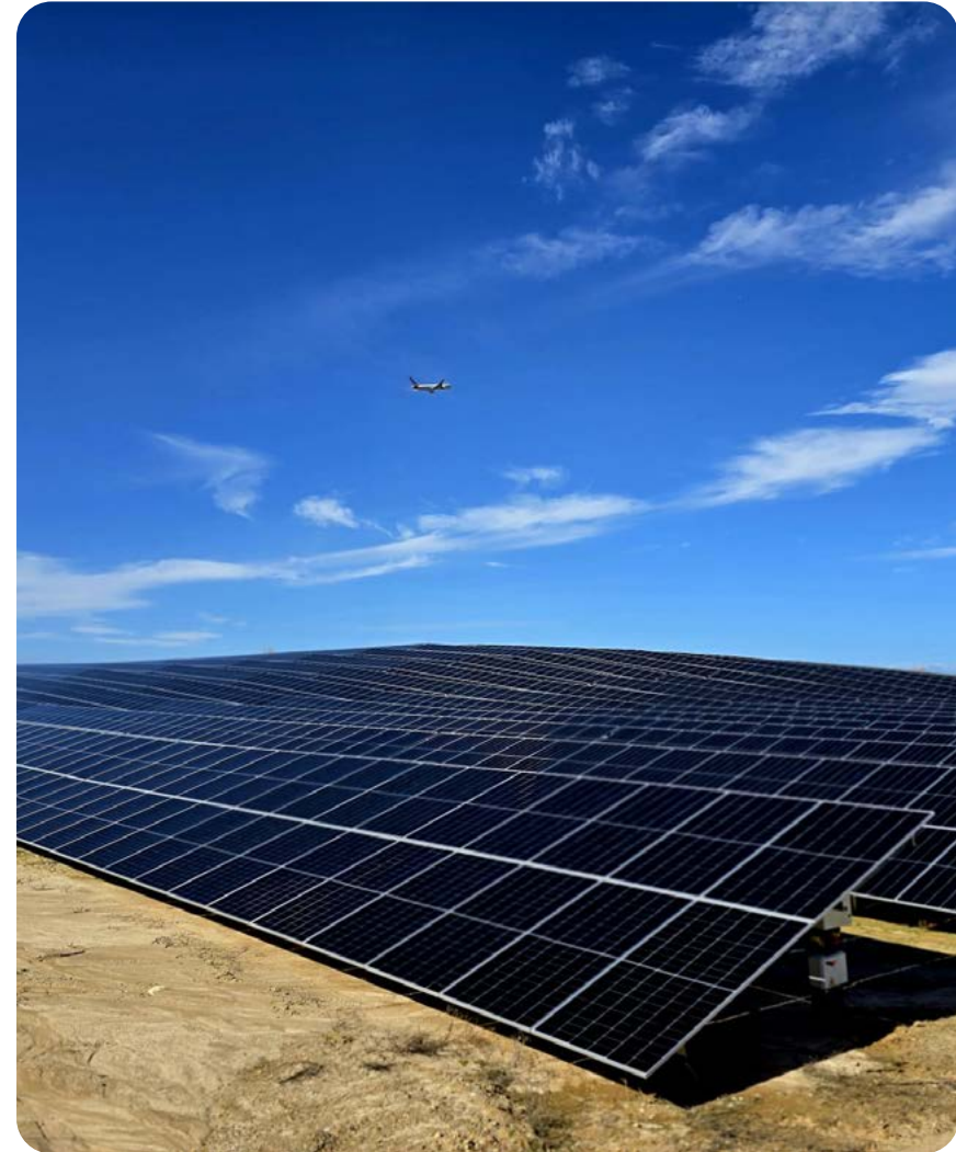
Photovoltaic plant at AS Madrid-Barajas Airport
